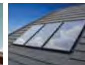
Solar thermal hot water
